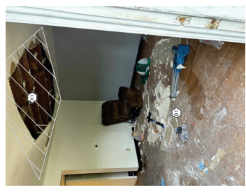
A VIEW OF GYPSUM BOARD/DEBRIS - LIVING ROOM
